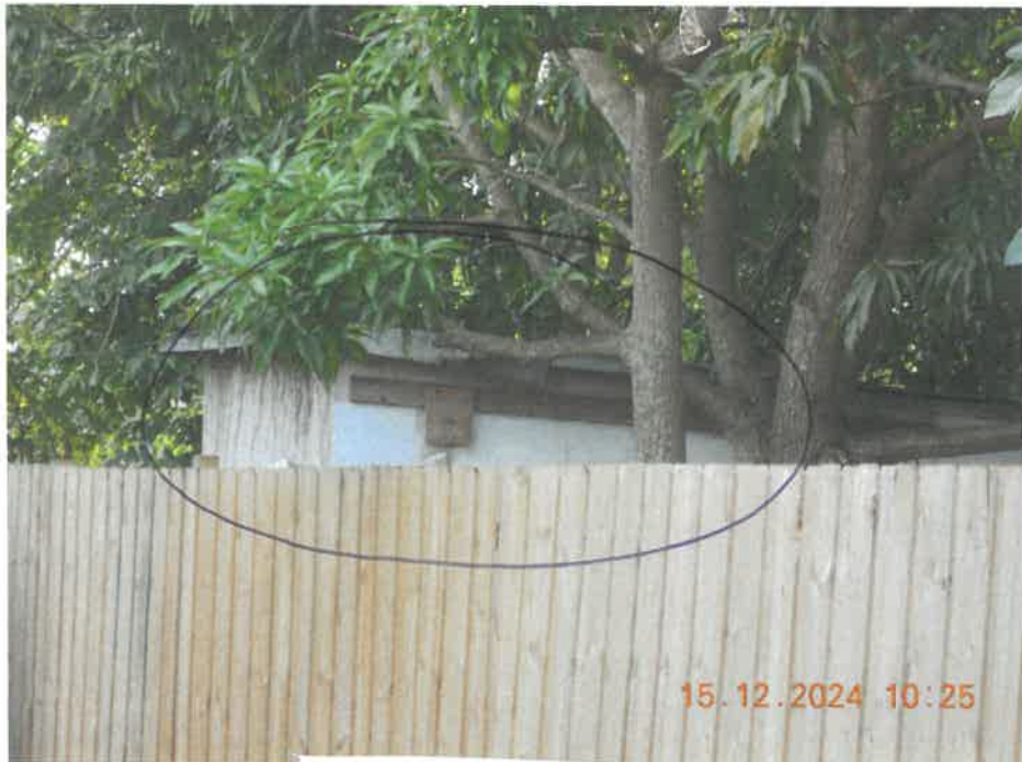
- Remove unpermitted structure.
