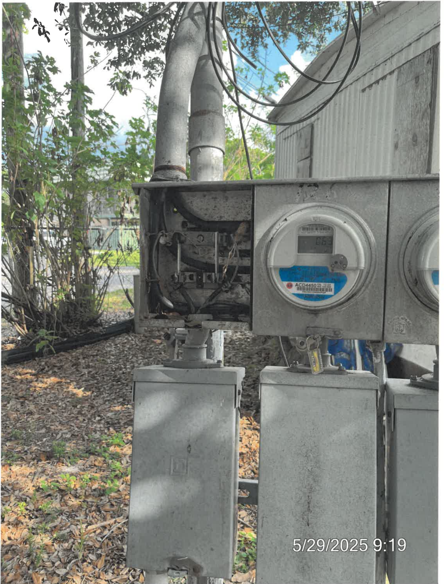
Code 2025-34 3206 Forest Hill Blvd (Section 10-31) FBC 116.1 UNSAFE ELECTRICIAN
